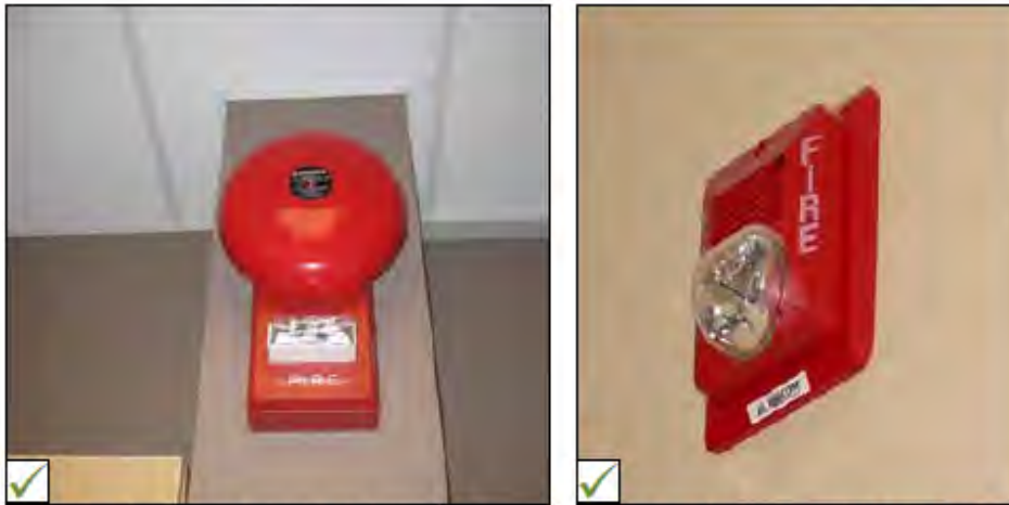
Example of combined visual and audible alarm signals. Public facilities should have both visual and audible fire alarm systems strategically located.
